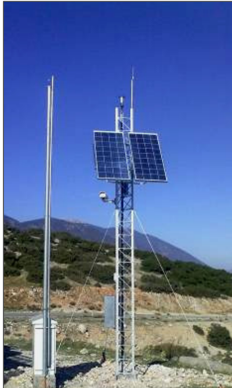
Meteorological Station (Greece)
