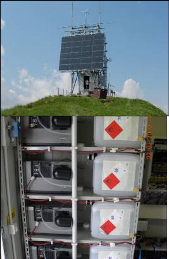
Repeater Stations EFOY Pro in Insulated Outdoor Box (Norway)
