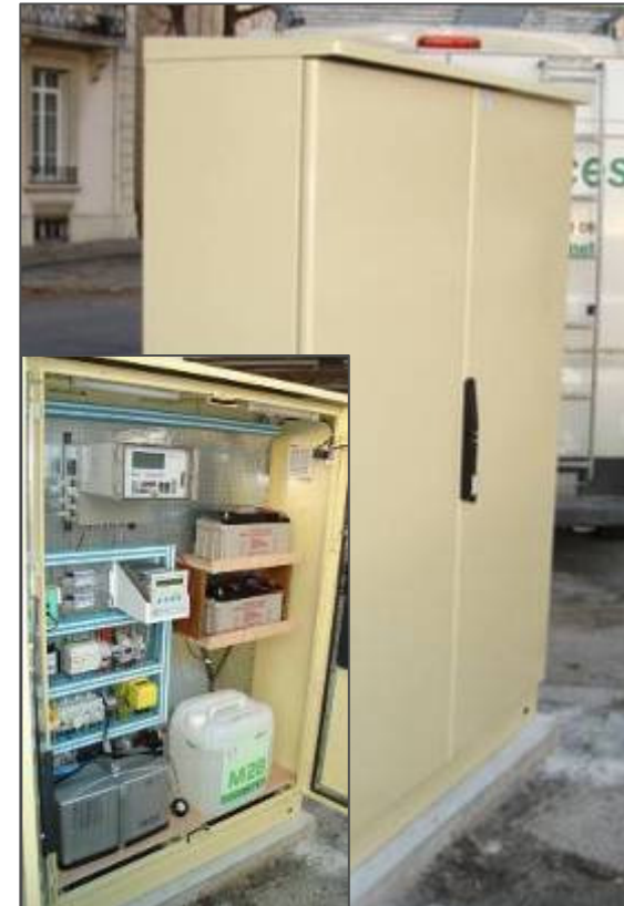
Water Flow and Gauge Measurement (France)
